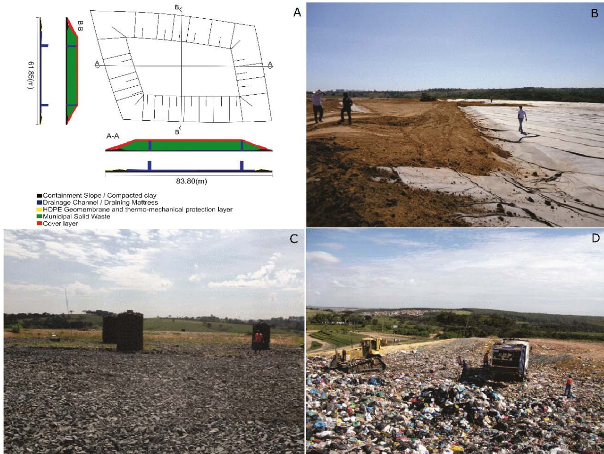
Figure 2 – Installation of the experimental cell. A) Implementation of the experimental cell at the MSW landfill Delta A. B) Geomembrane installation in the beginning of the implementation of the experimental cell. C) Drainage system completed. D) Compression of the MSW within the experimental cell. (Extracted from Benatti et al., 2013).
